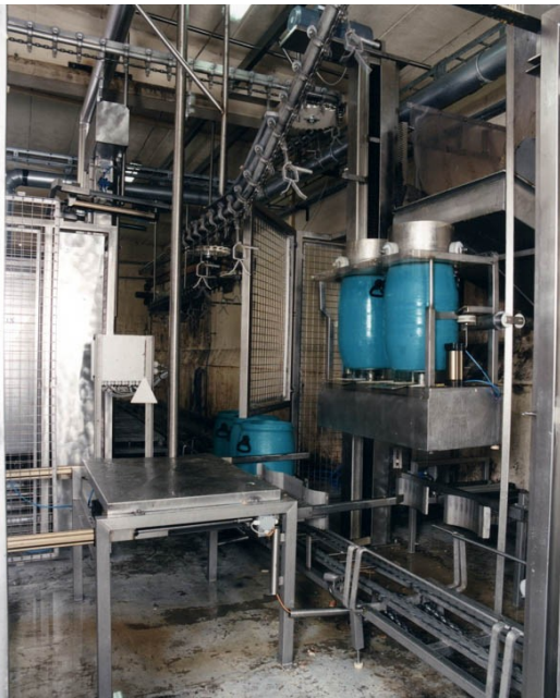
EMPTY AND IN-FEED UNIT
